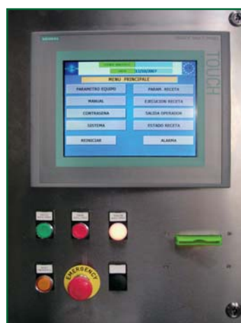
Touch Screen controllo remoto Remote Touch Screen control
